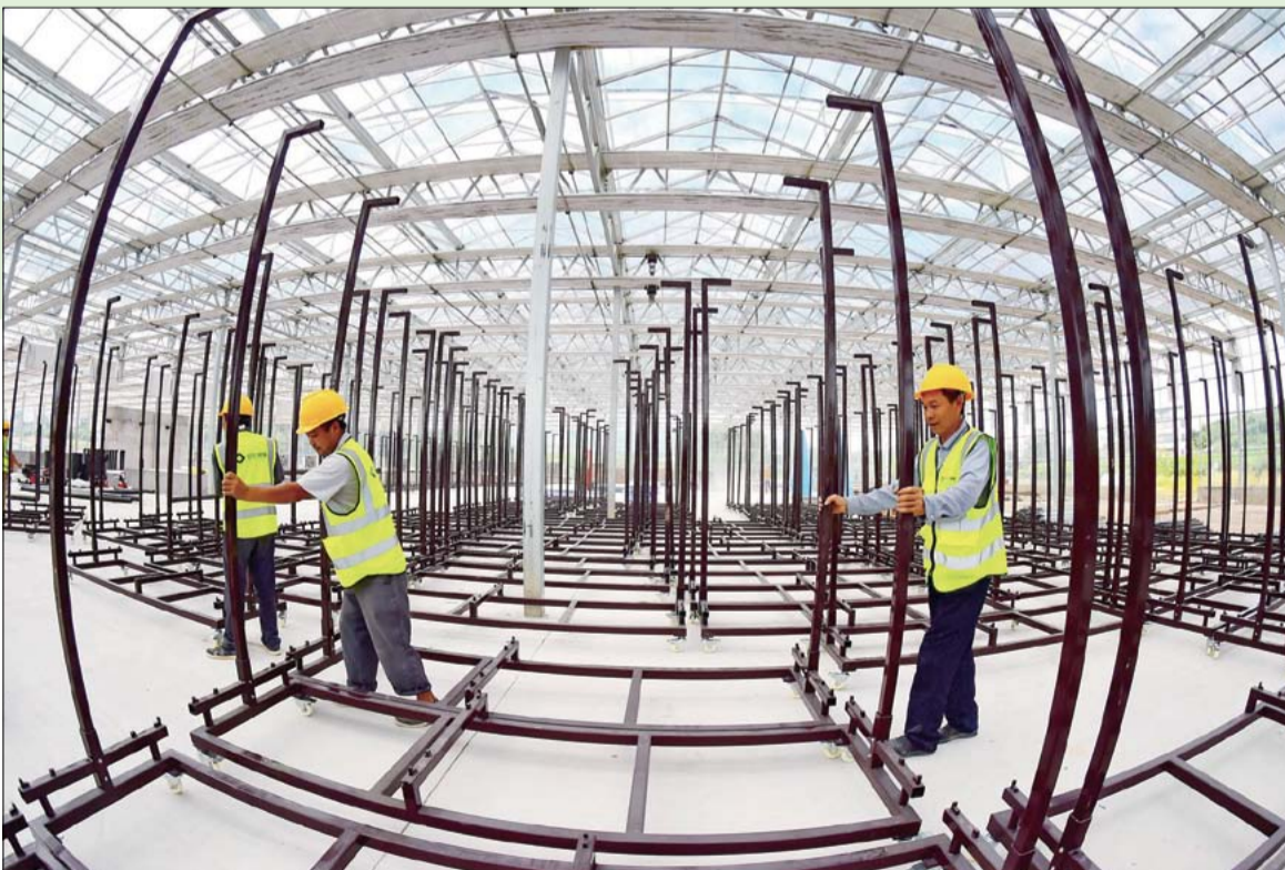
Workers set up a greenhouse for the aquaponic system which integrates fish raising and soil-less growing of plants in Ganzhou City, Jiangxi Province.
